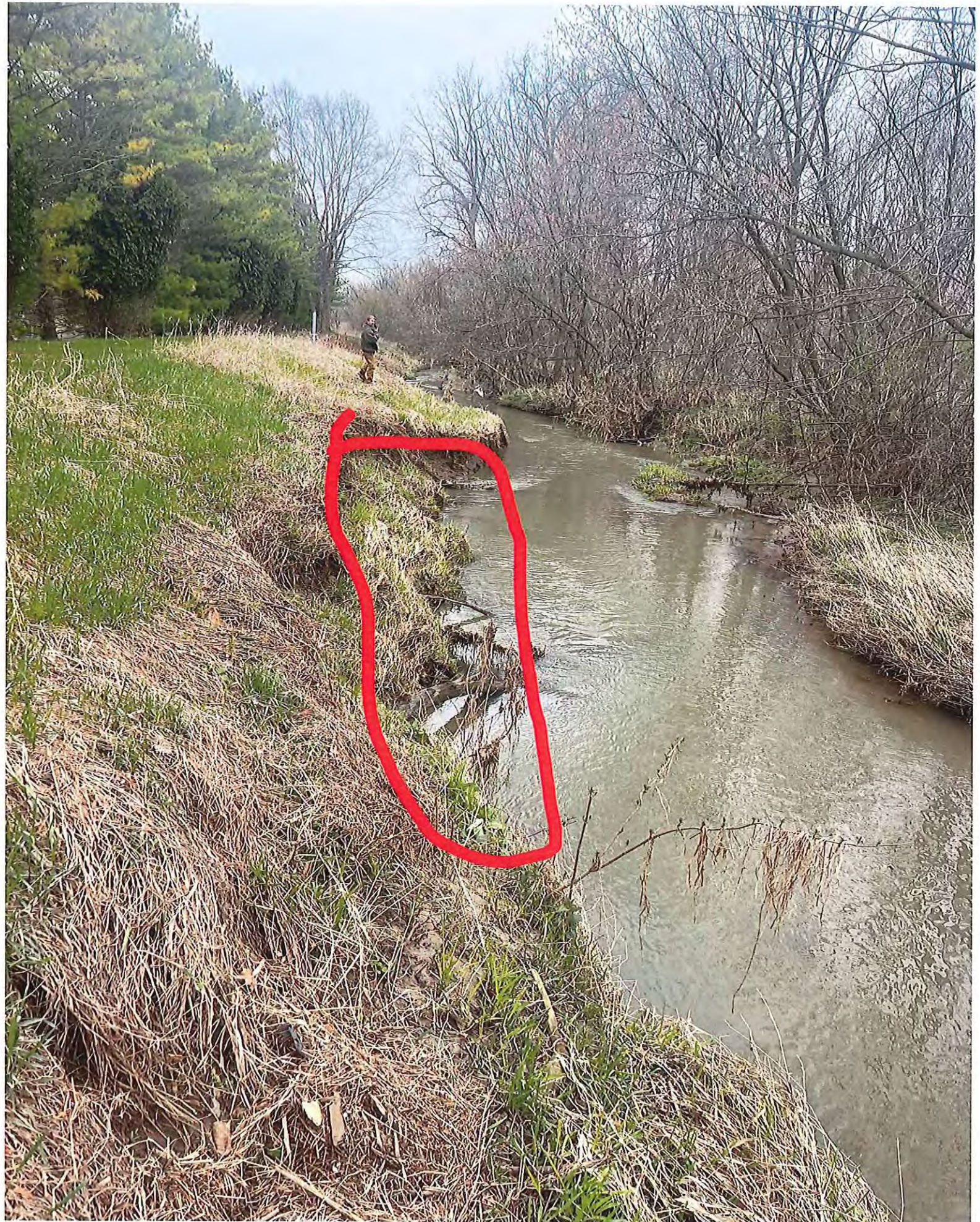
SITE J Project #25-006 Horn Ditch Brushing and Maintenance Project: erosion SITE J
