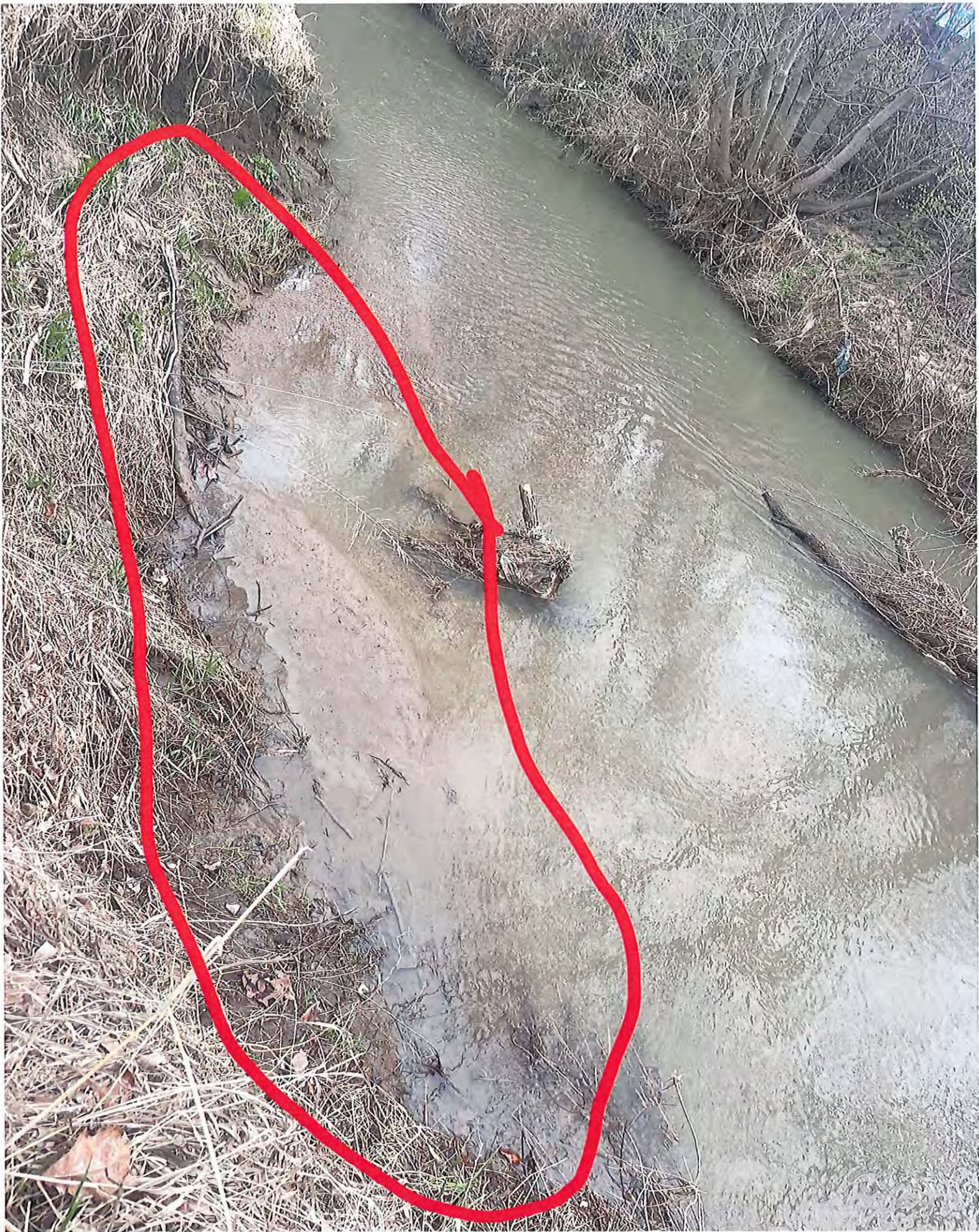
SITE C Project #25-006 Horn Ditch Brushing and Maintenance Project: erosion SITE C
