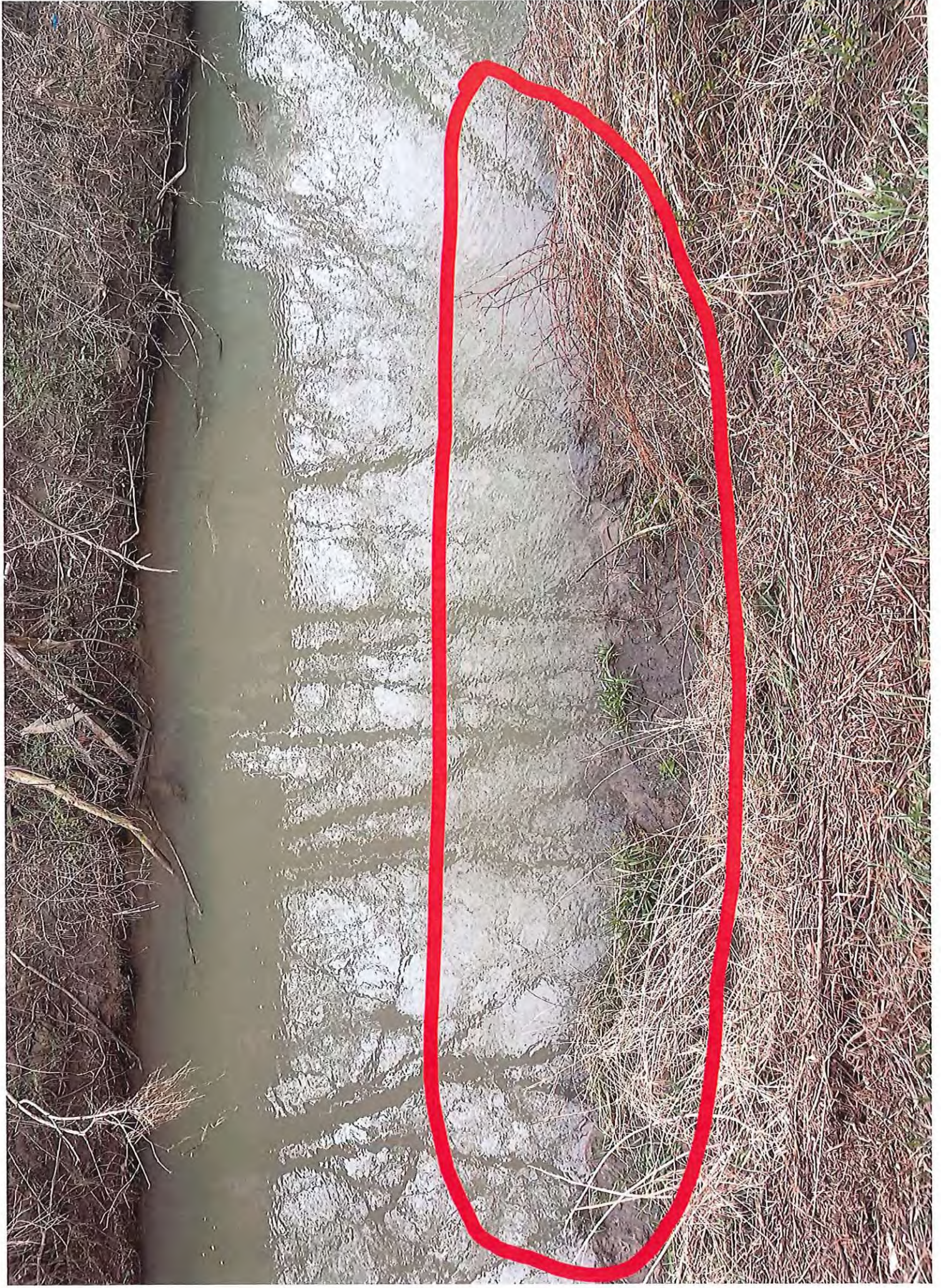
SITE B Project #25-006 Horn Ditch Brushing and Maintenance Project: erosion SITE B
