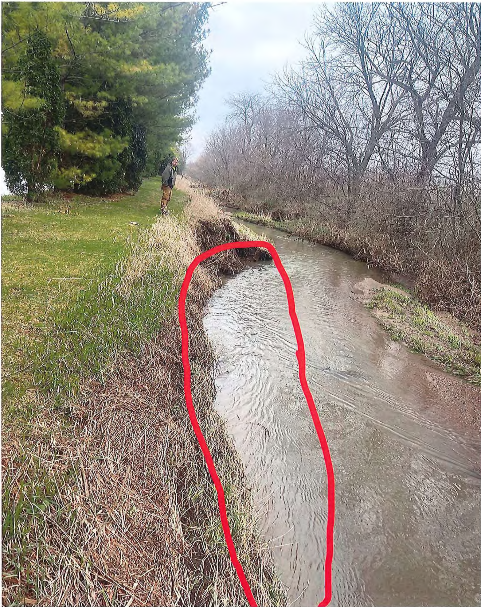
SITE F Project #25-006 Horn Ditch Brushing and Maintenance Project: erosion SITE F
