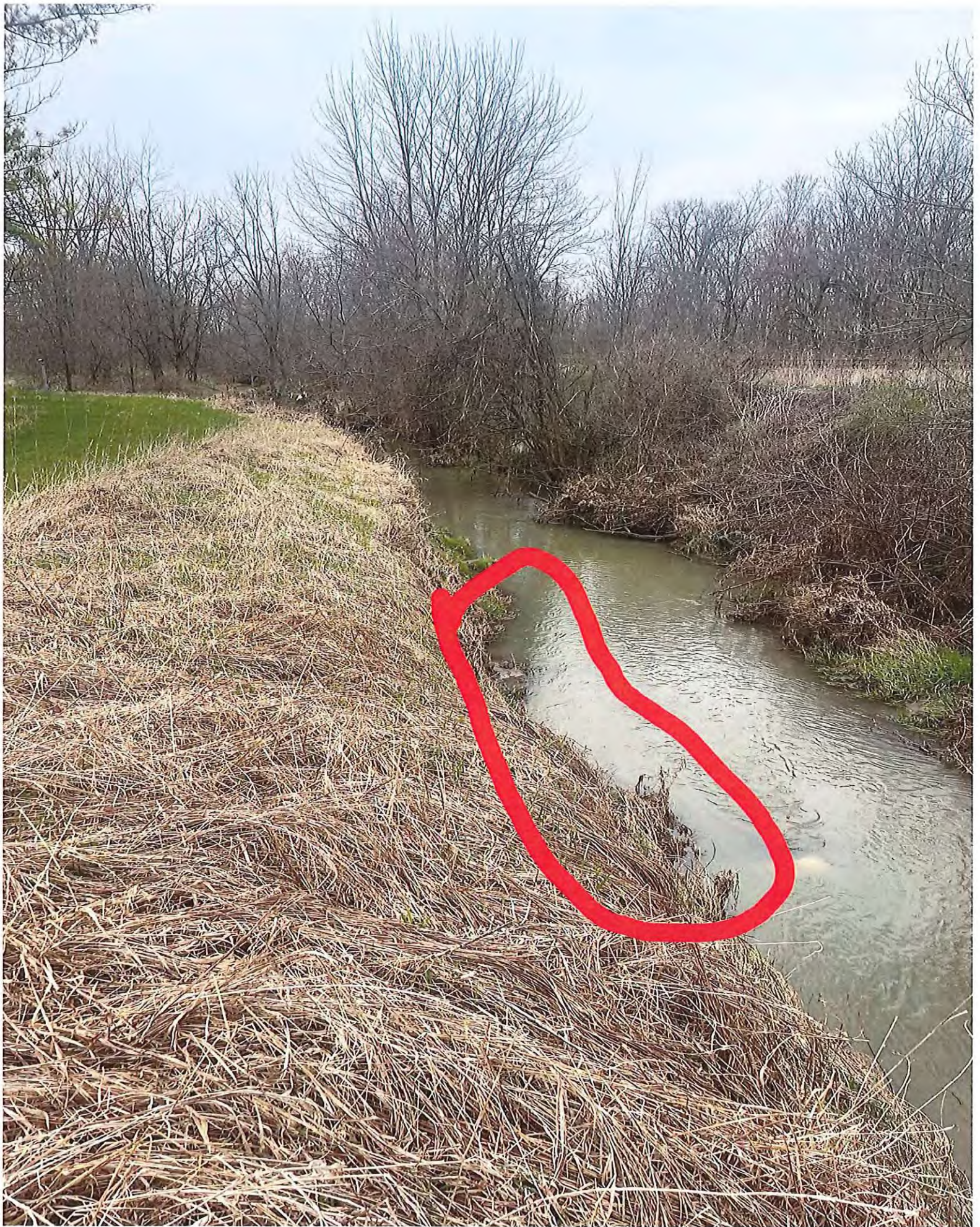
SITE L Project #25-006 Horn Ditch Brushing and Maintenance Project: erosion SITE L
