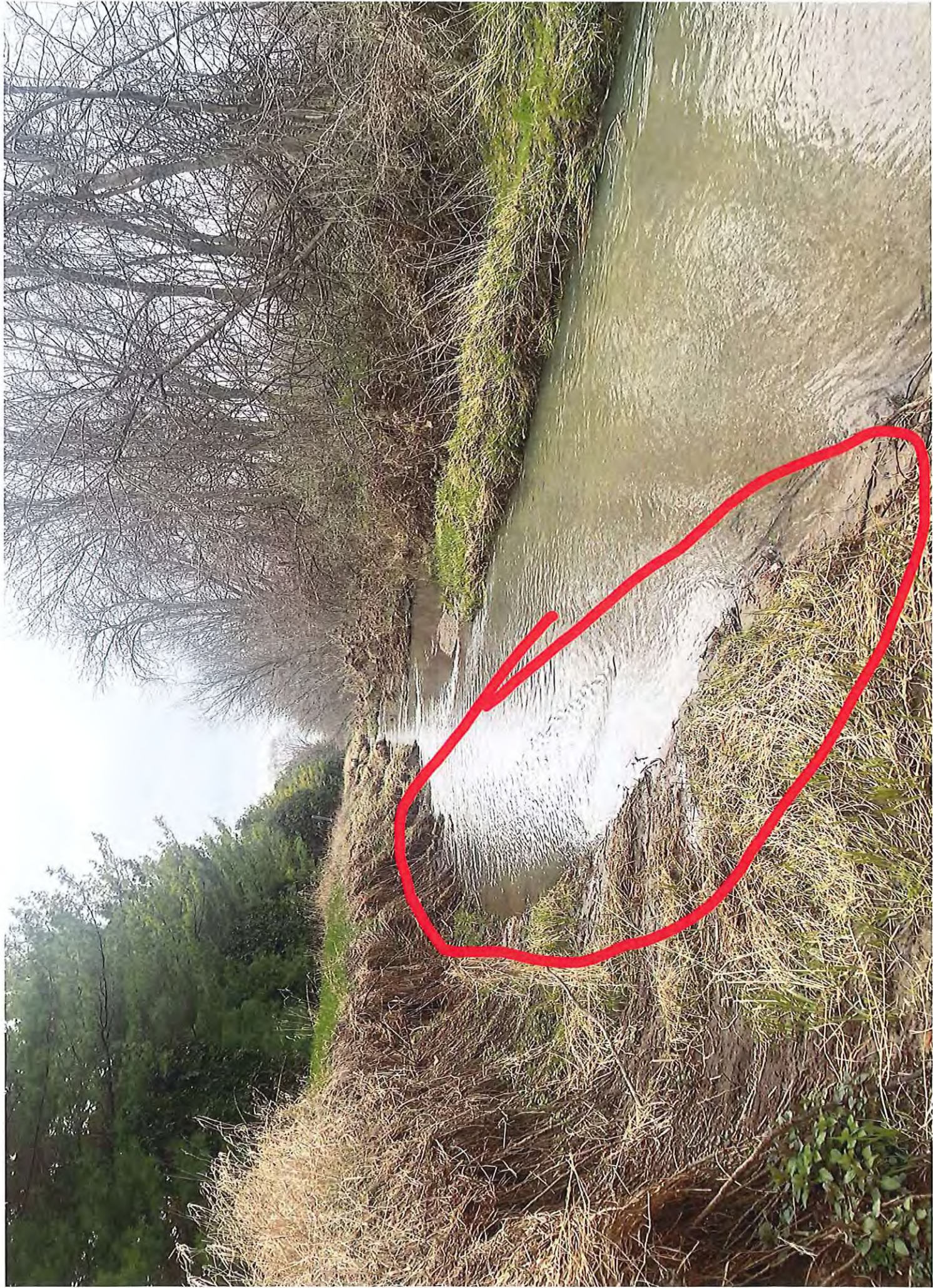
SITE G Project #25-006 Horn Ditch Brushing and Maintenance Project: erosion SITE G
