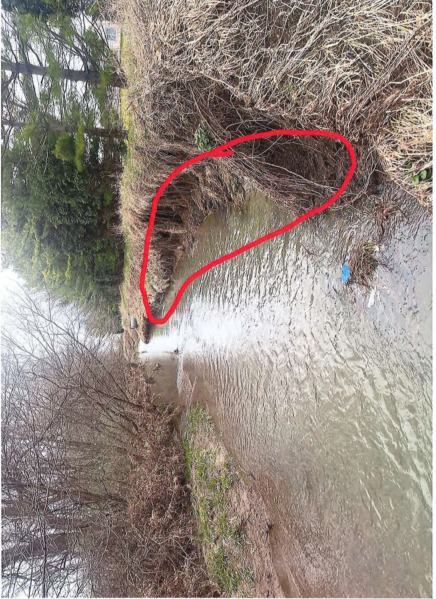
SITE F Project #25-006 Horn Ditch Brushing and Maintenance Project: erosion SITE F
