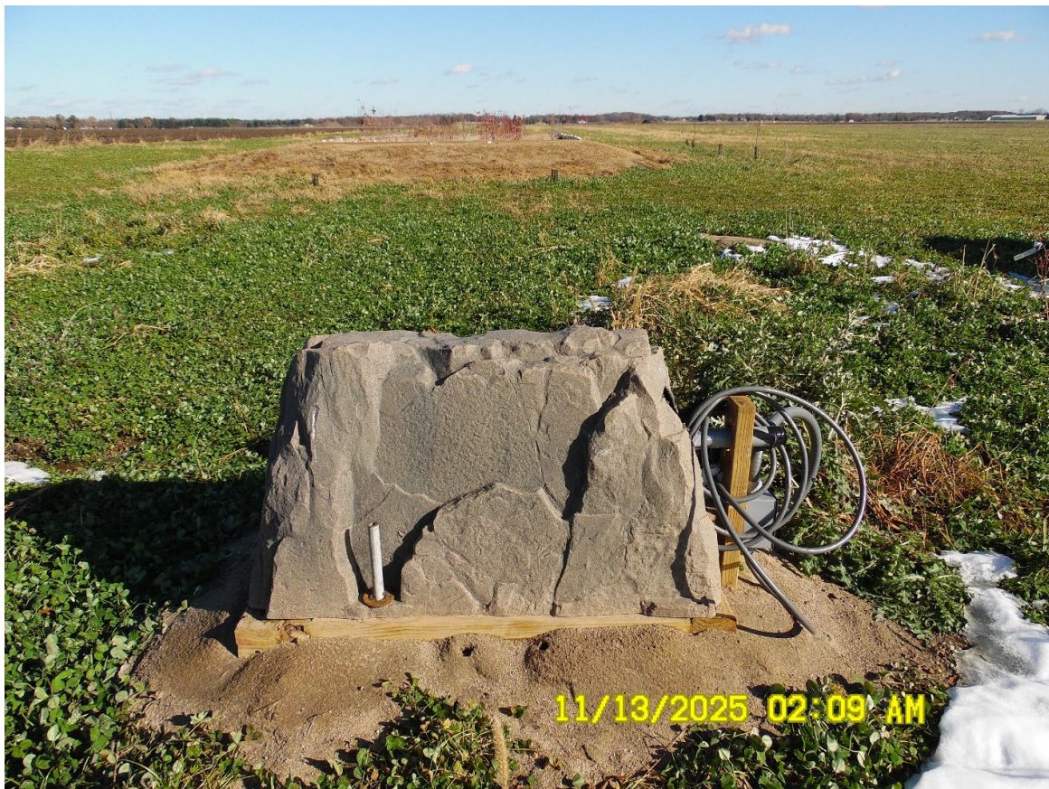
Looking east at well pump
