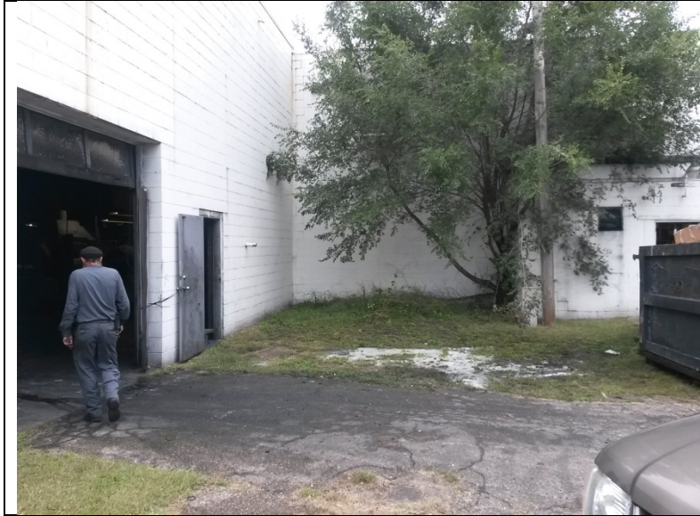
Impacted area by dumped slab dip
