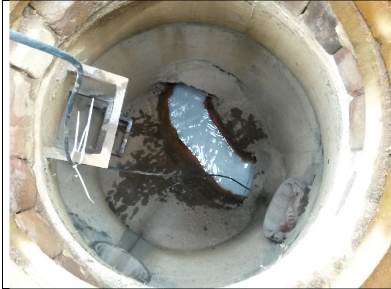
City of Goshen Stormwater Manhole 507-3358 seen change white while installing a flow meter
