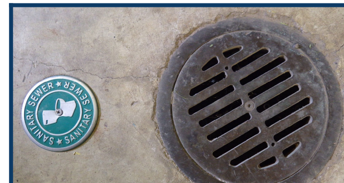
Interior floor drains should be marked with a green sanitary medallion.
