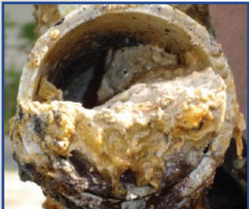
A clogged pipe caused by the dumping of F.O.G. down the drain. Photo Credit: City of Elkhart
