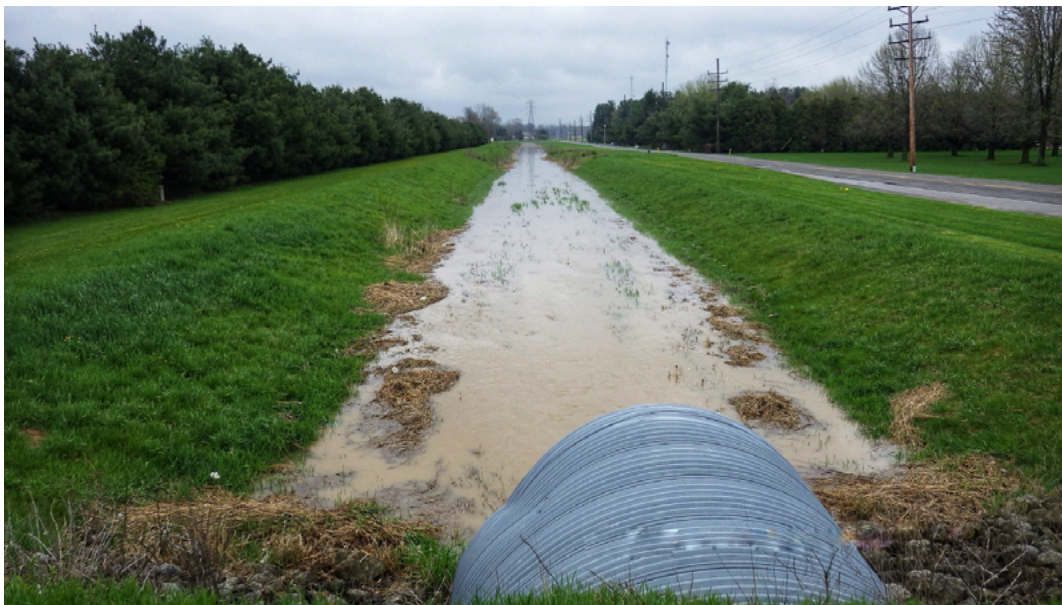
Figure 32: Looking east from Northstone Road at sediment-laden stormwater flowing through the County Road 36 Diversion Ditch during a May 2018 rain event.
