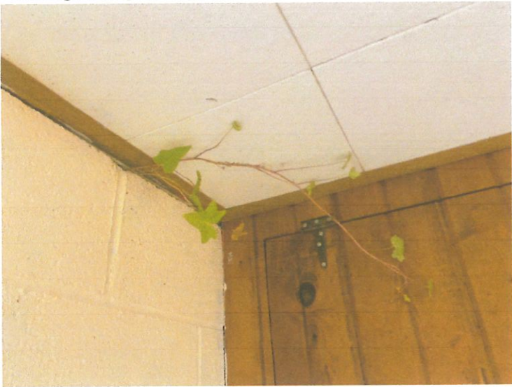
Trees growing through basement walls
