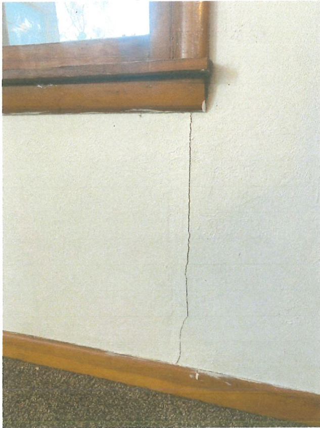
Cracked walls throughout home
