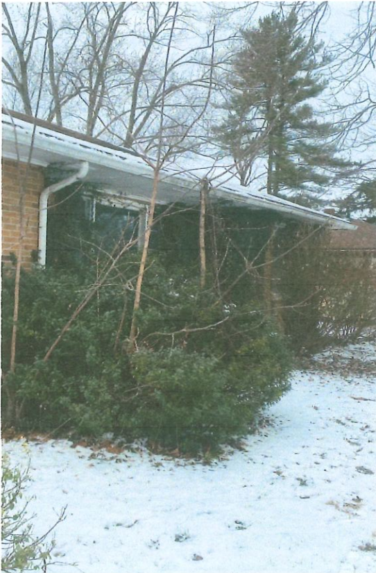
Gutters have not been cared for, and need replaced
