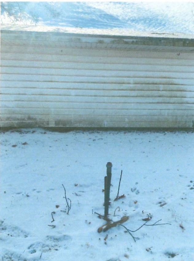
Exterior of home needs power washed
