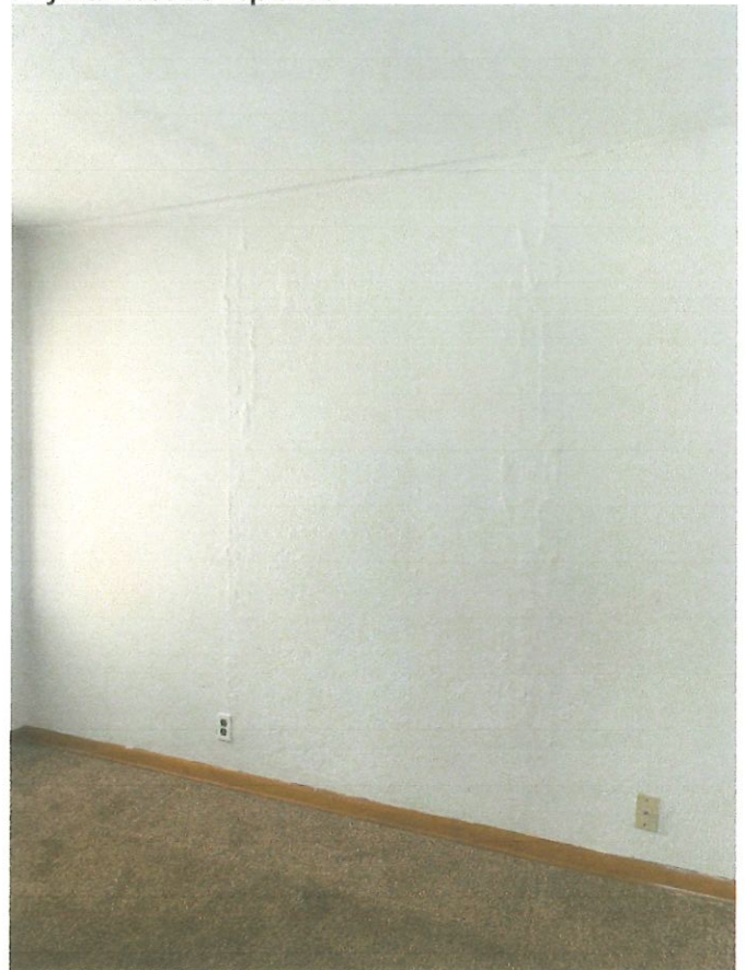
Drywall needs repaired
