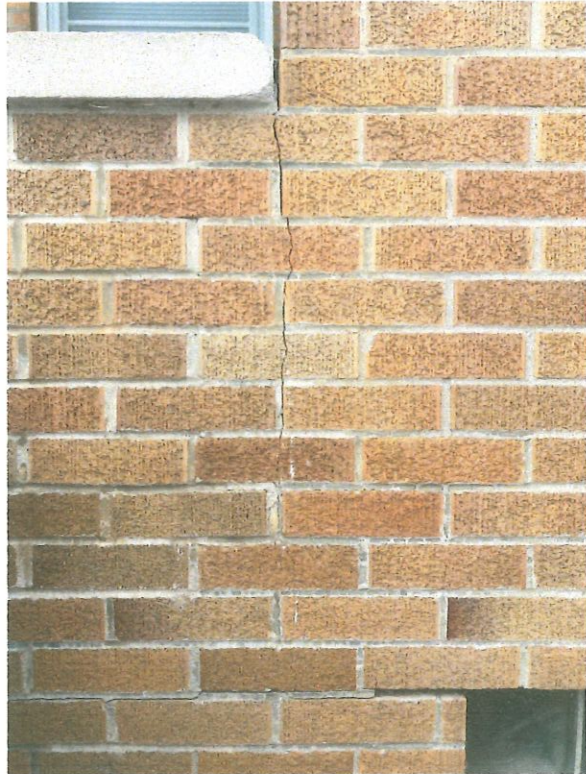
Tuck Pointing needed on exterior brick
