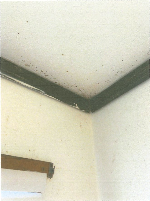
Mold and damaged trim
