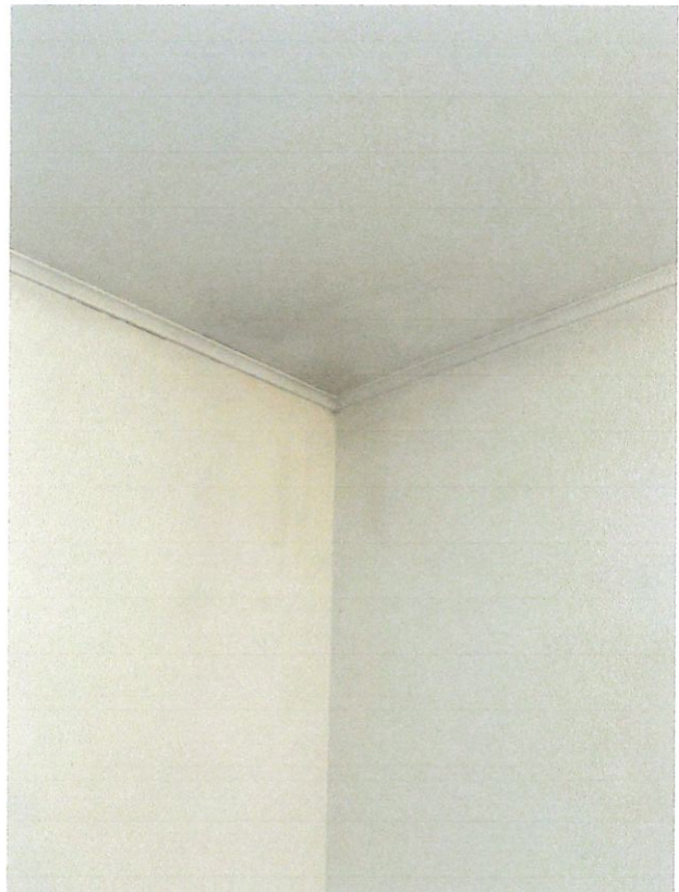
Evidence of mold/water damage needs inspected/ repaired
