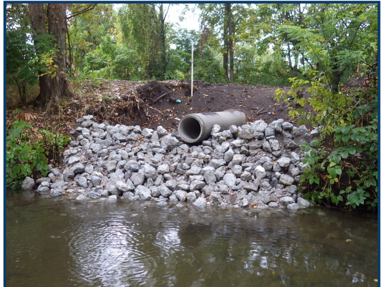
The Goshen Water & Sewer Department repairs or replaces damaged storm sewer outlet pipes.
