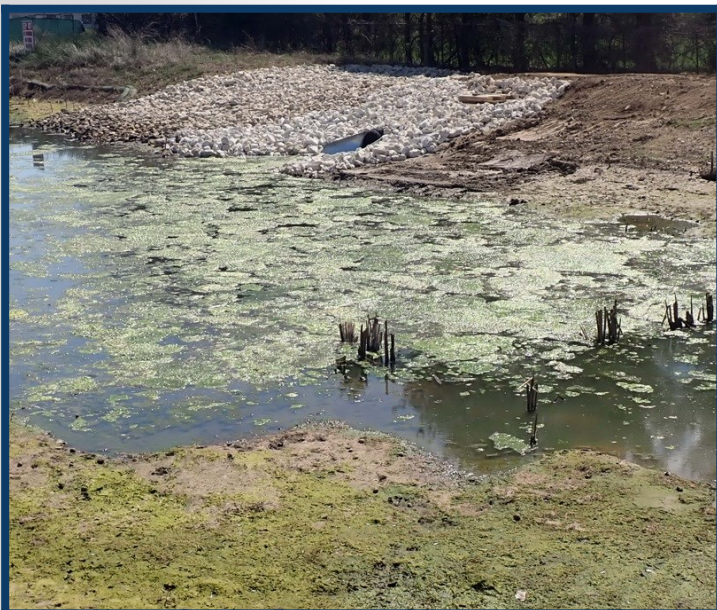
Detention Basin showing the release structure for water to flow from pond.
