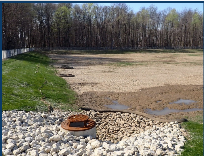
Outflow structure and drywells in Basin #1, at the south end of the project.
