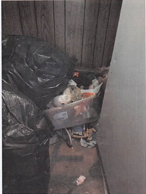
Trash, junk, debris in kitchen, Apt. 3.
