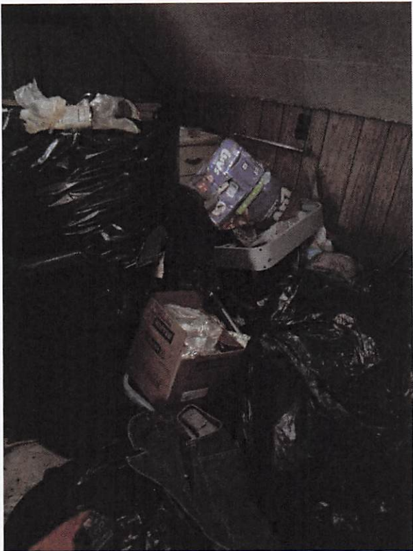
Trash, junk, debris in kitchen, Apt. 3.
