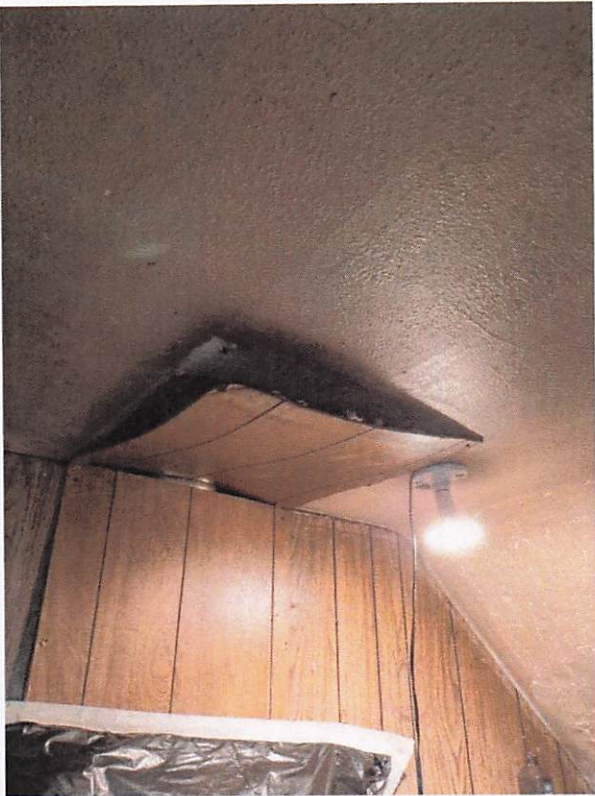
Ceiling in disrepair, Apt. 3.
