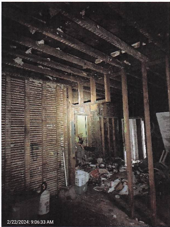
2/22/2024: 9:06:33 AM Walls, ceiling in disrepair, Apt. 3.
