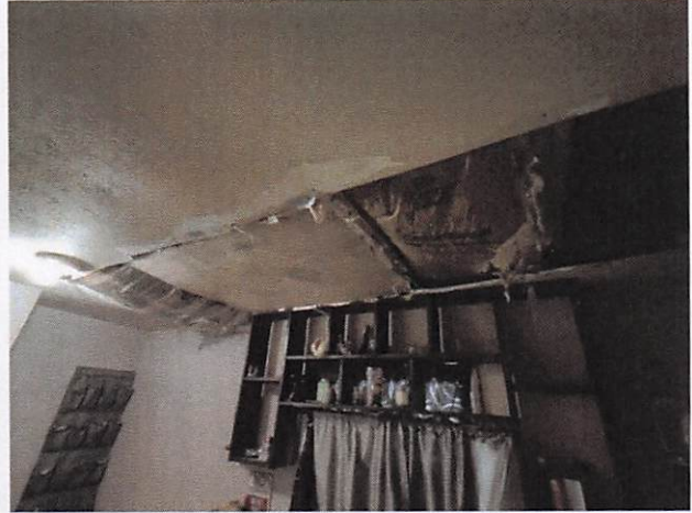
Ceiling in disrepair, Apt. 2
