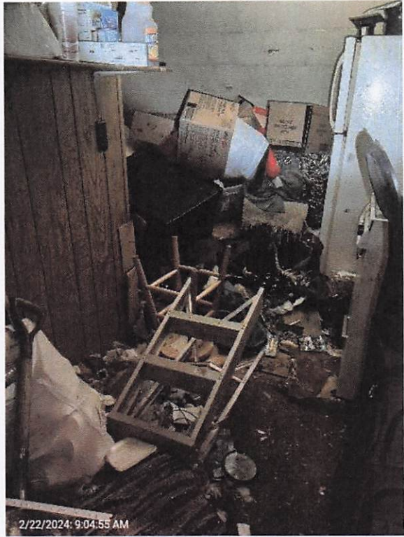
Trash, junk, debris in kitchen, Apt. 3.
