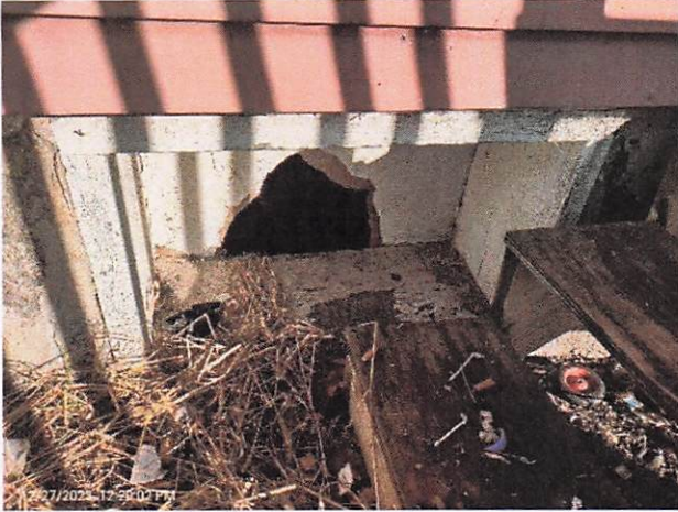
Hole in exterior wall.
