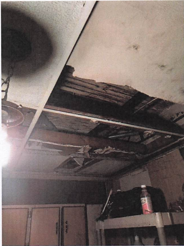
Collapsing ceiling, Apt. 2
