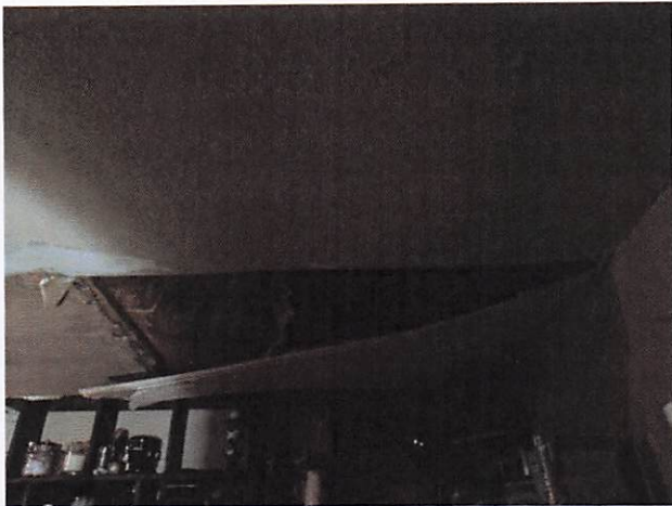
Collapsing ceiling, Apt. 2
