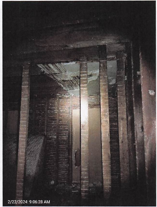
2/22/2024: 9:06:28 AM Walls, ceilings in disrepair, Apt. 3
