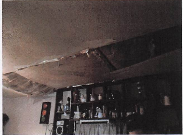
Collapsing ceiling, Apt. 2
